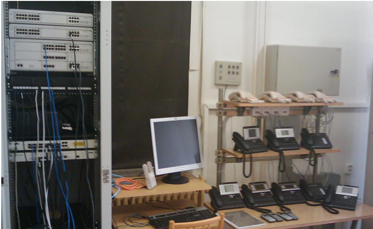
Figure 3. The Alcatel-Lucent OmniPCX Enterprise workplace.
